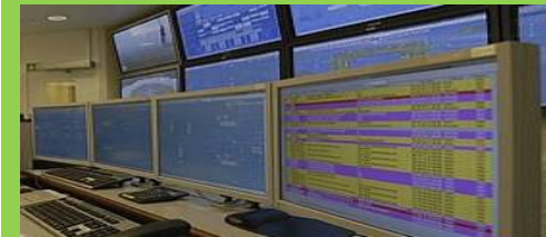
Asset control room
